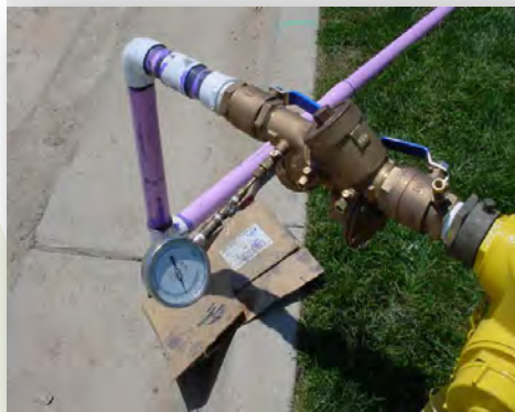
Highline with Potable
